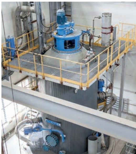
The 30 m high steam-phase digester was installed first and the building was erected around it. ▼
