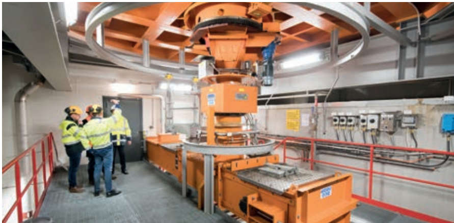
▲ Shown is a fuel discharging system at the bottom of one of the day silos. The plant is equipped with two such systems for redundancy reasons.
