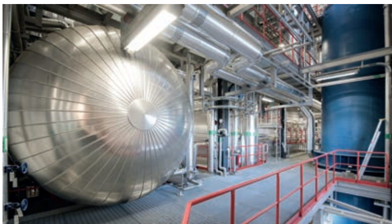
▲ The feedwater tank in the ANDRITZ BFB boiler.
