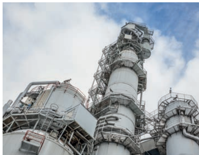
◀ ANDRITZ modernized several areas of the softwood fiberline at Kymi as part of the KYMI-700 project.
