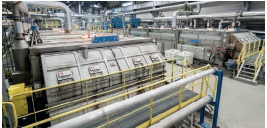
▲ Vacuum table washers in new ANDRITZ advanced Green Liquor plant.
