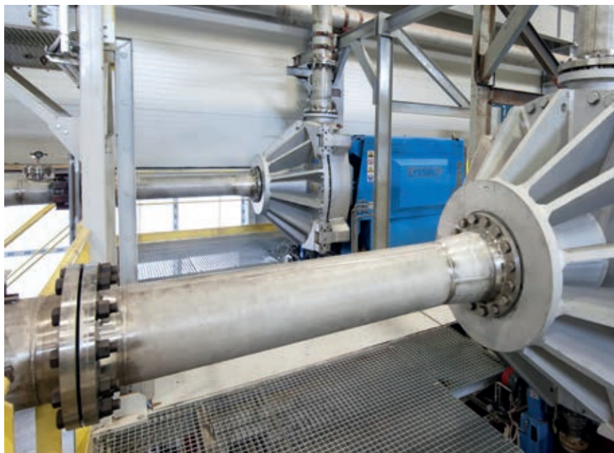
▼ MC blowline refiners after the digester.
