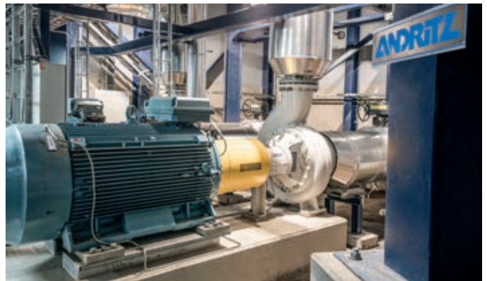
Water recirculation pump for flue gas condensing system. ▶
